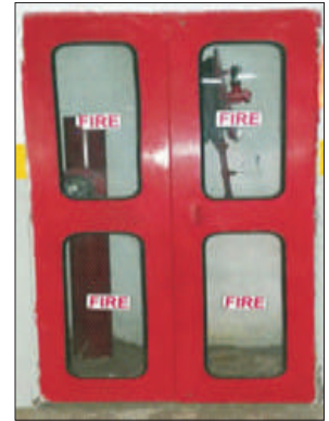
Fire Hydrant Cabinet
