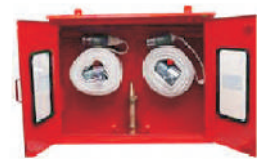
Fire Hose Box
